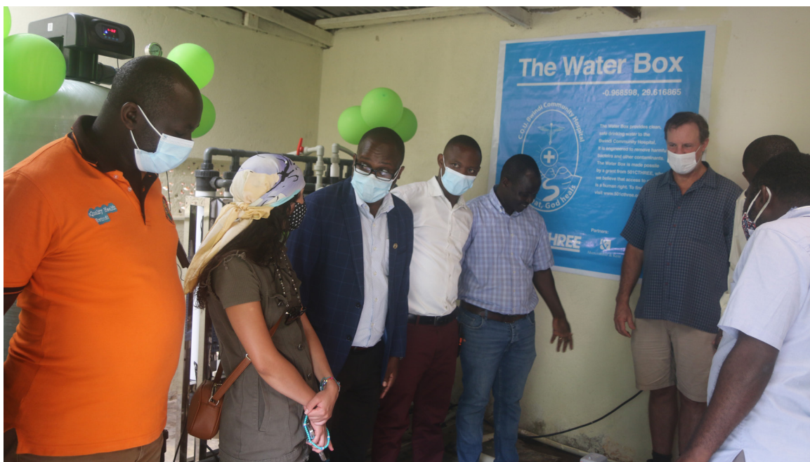
Commissioning of the Tiva water filtration plant donated by AKP
