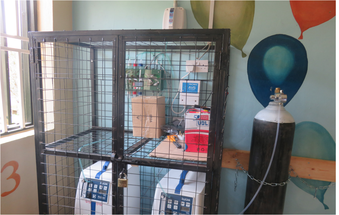
Mini oxygen plant installed for the new borns by FreO2
